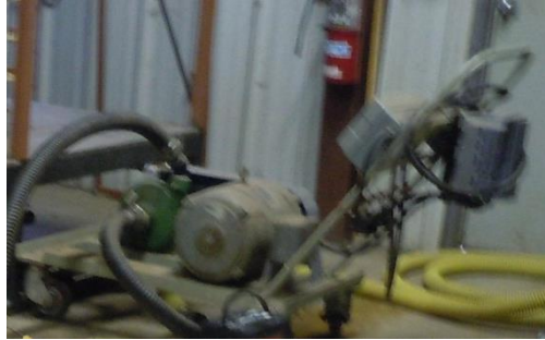
Figure 13. Primary system 2" centrifugal pump with 10hp electric motor.
