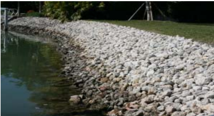
Figure 7: Riprap along a coastal shoreline in Florida (Garland & Garland, 2014).
